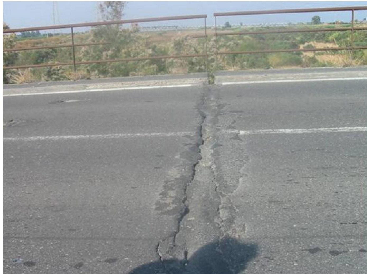
Disrupted bridge joints
