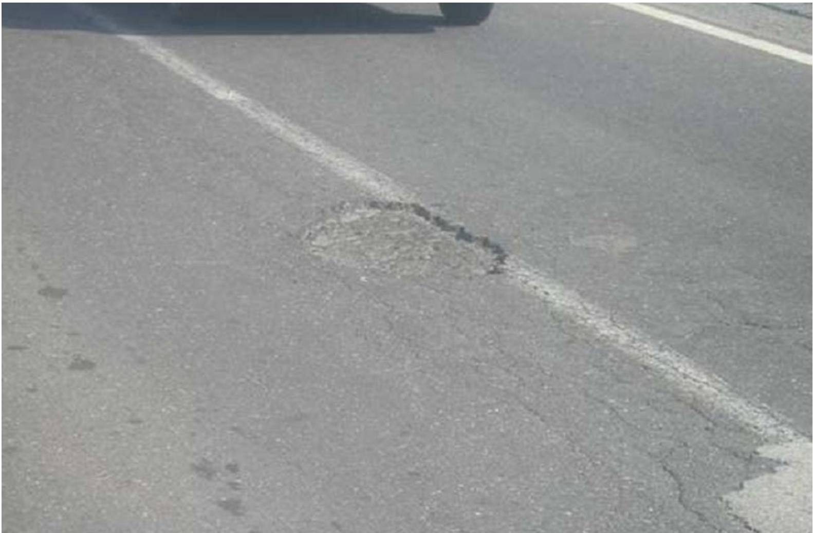
Superficial pothole on tangent
