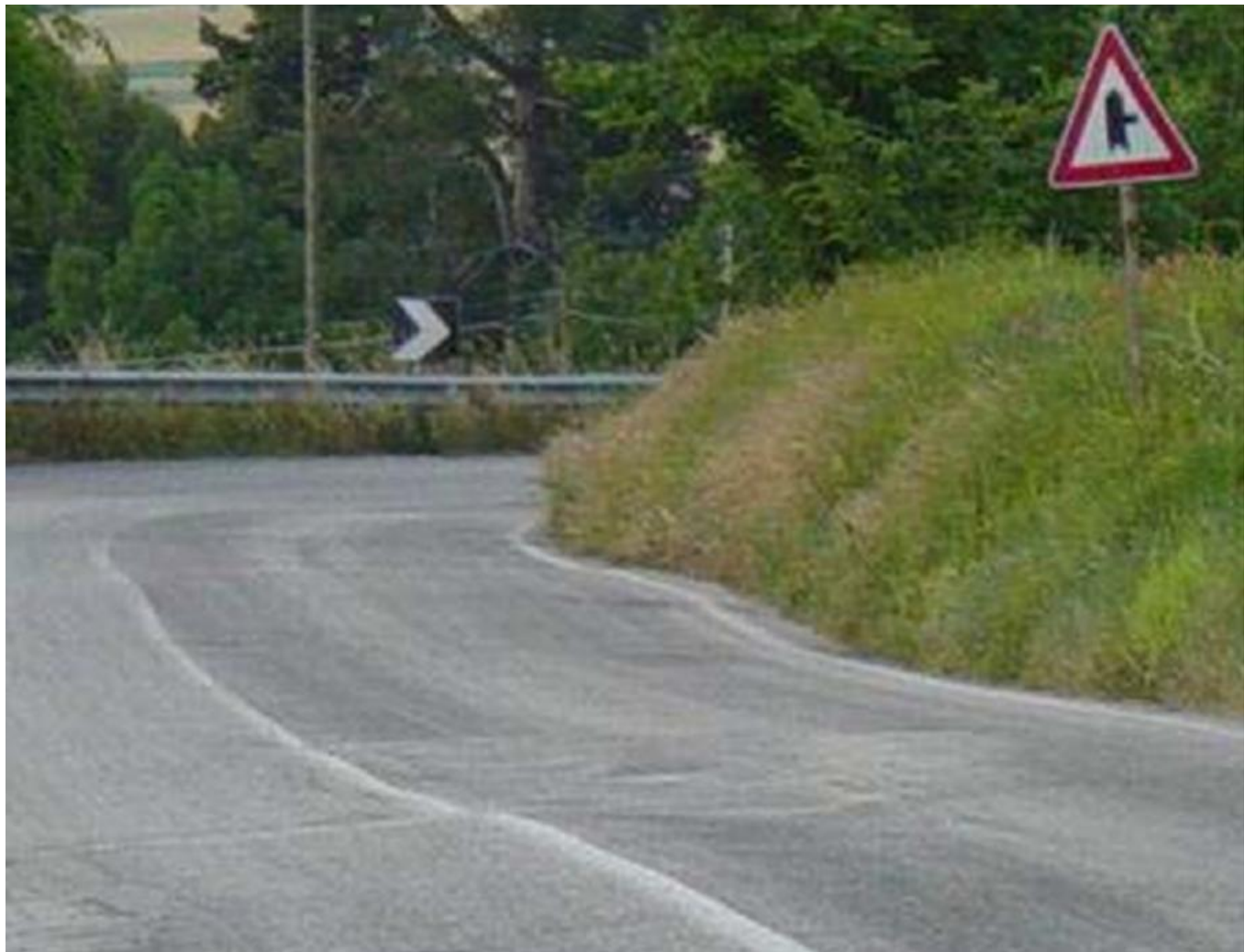
Shoving on curve approach
