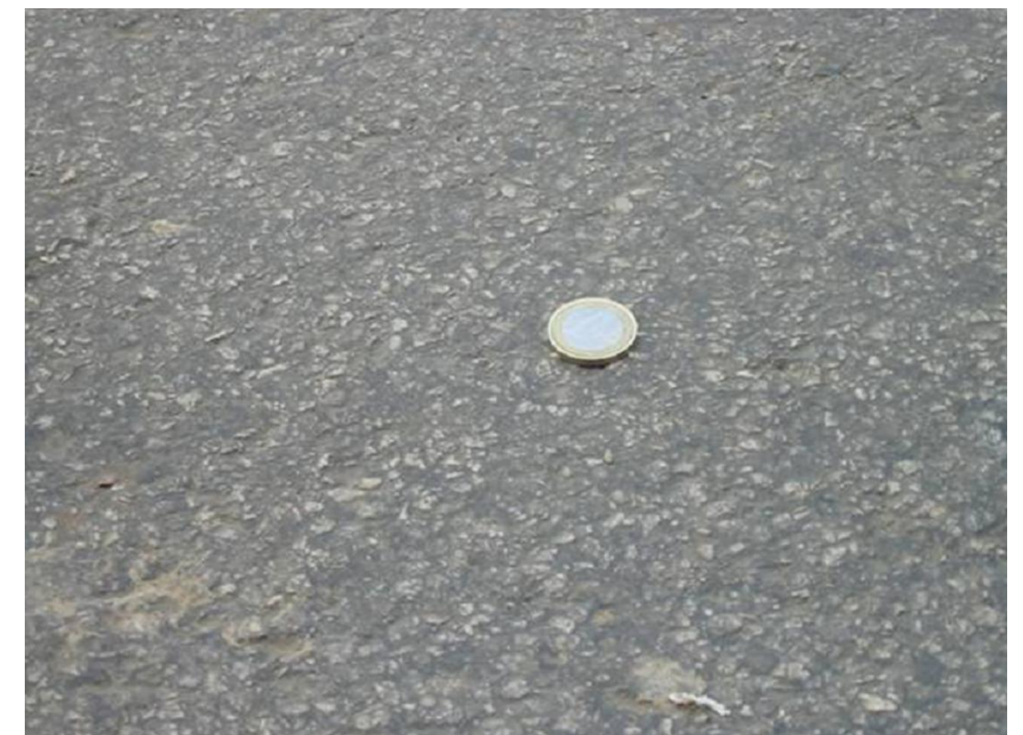
Low macrotexture and bleeding
